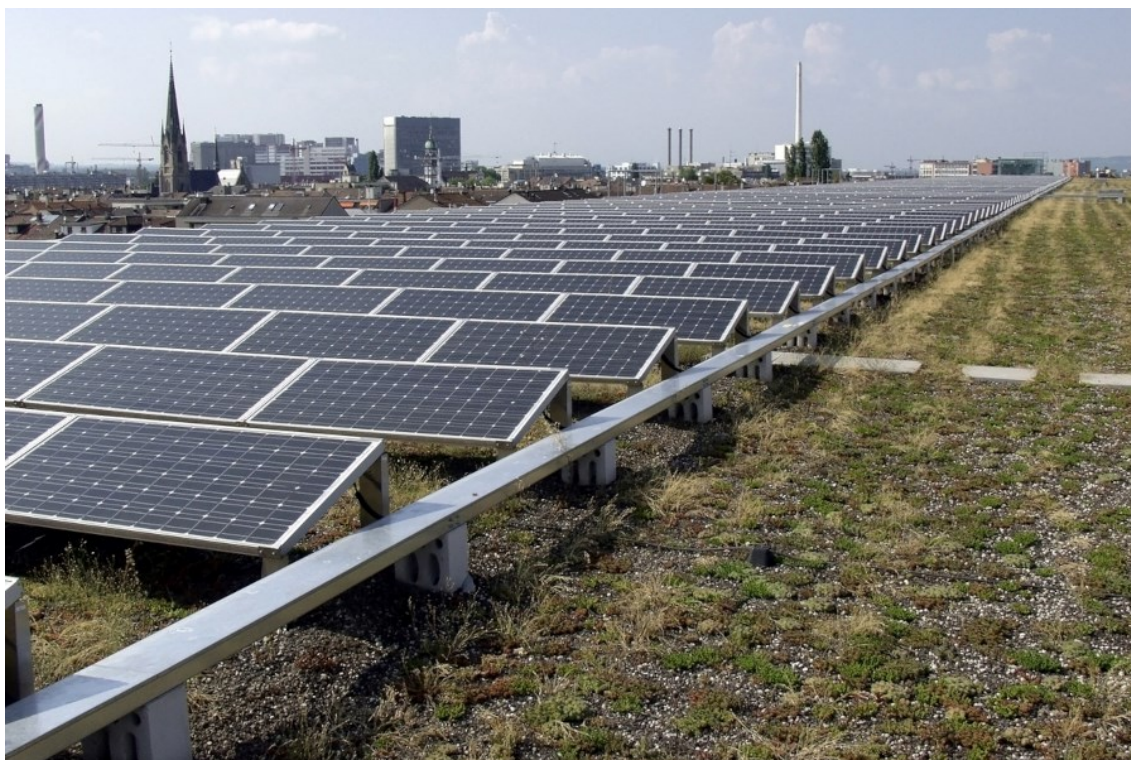
Messe Basel | Photovoltaikanlage
