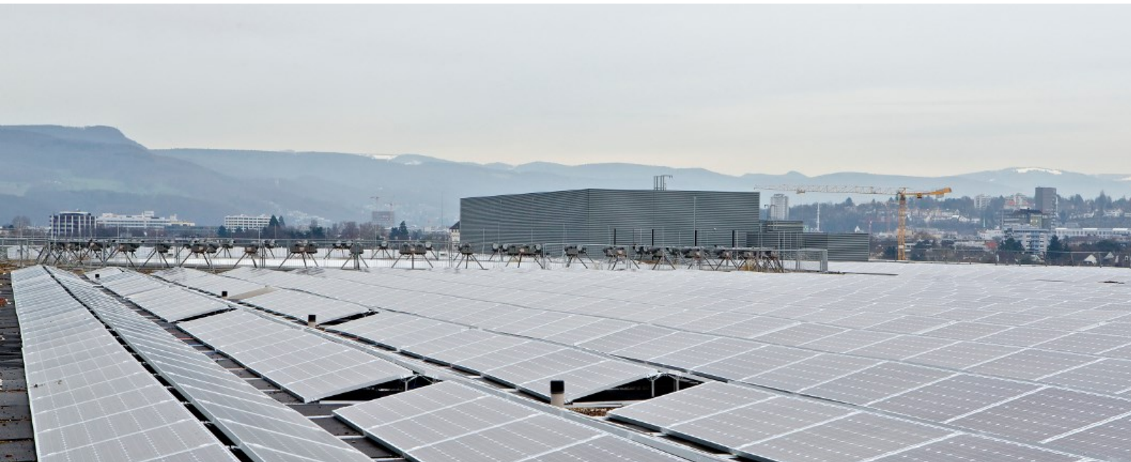
Installations photovoltaïques Messe Basel, Halle 1
