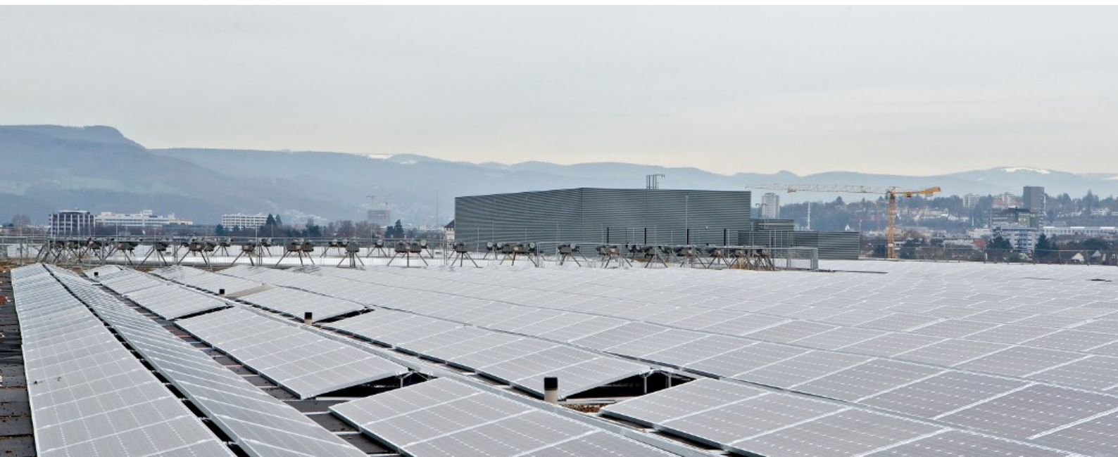
Photovoltaik-Anlage Messe Basel, Halle 1
