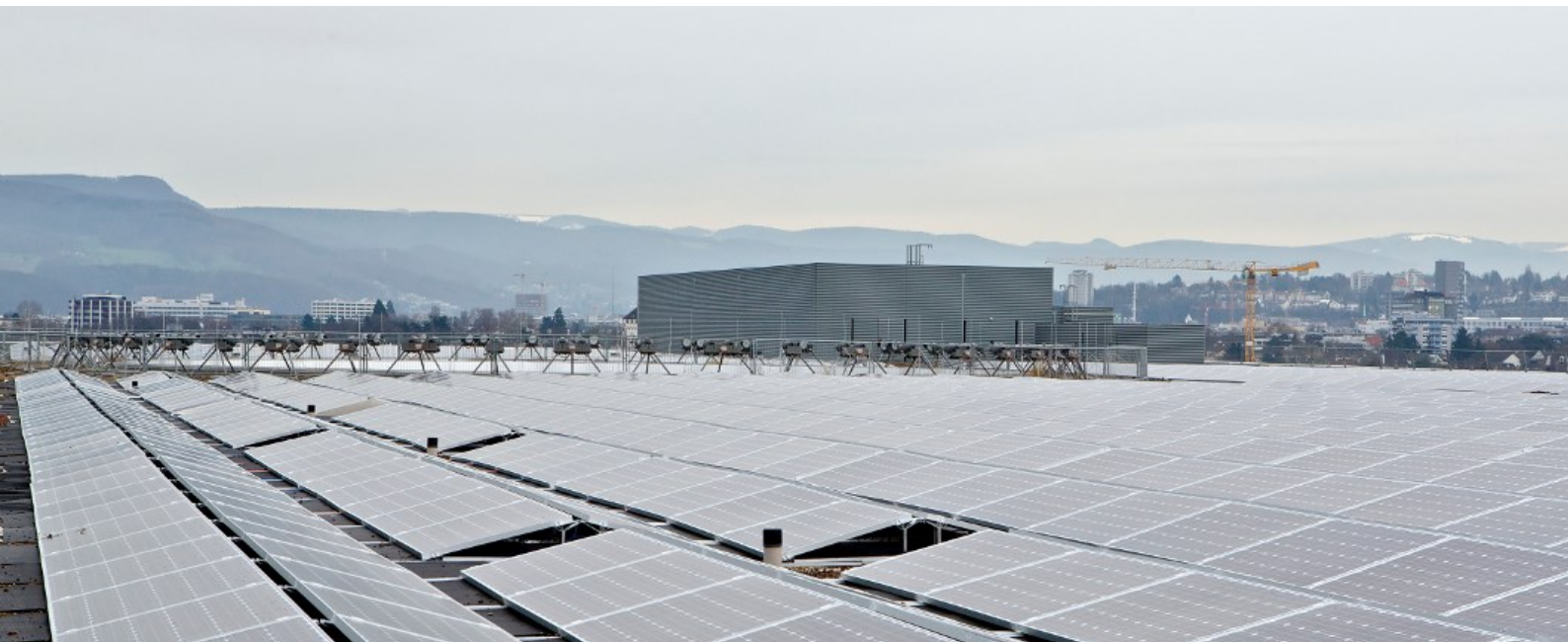
Photovoltaic system Messe Basel, Hall 1
